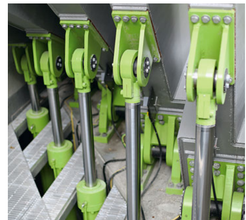
Hydraulic cylinders for raising and lowering the bridge
