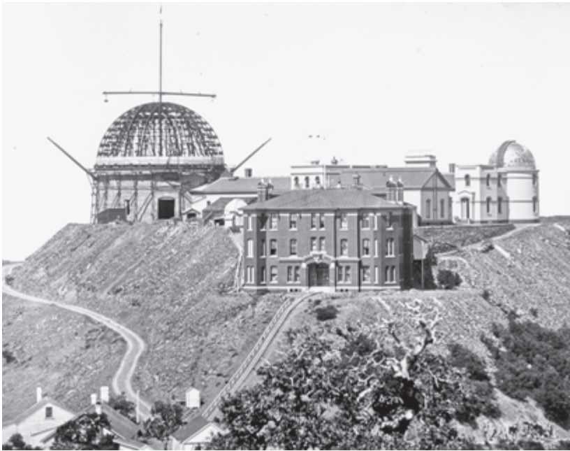
38. The Lick Observatory on Mount Hamilton, photographed during construction of the main dome by Warner & Swasey (completed in 1887). In 1891 Michelson undertook interferometric measures of the diameter of Jupiter's moons using adjustable slits placed over the objective of the twelve-inch equatorial telescope in the dome to the right. Lick Observatory Archives, courtesy AIP Emilio Segre Visual Archives.
