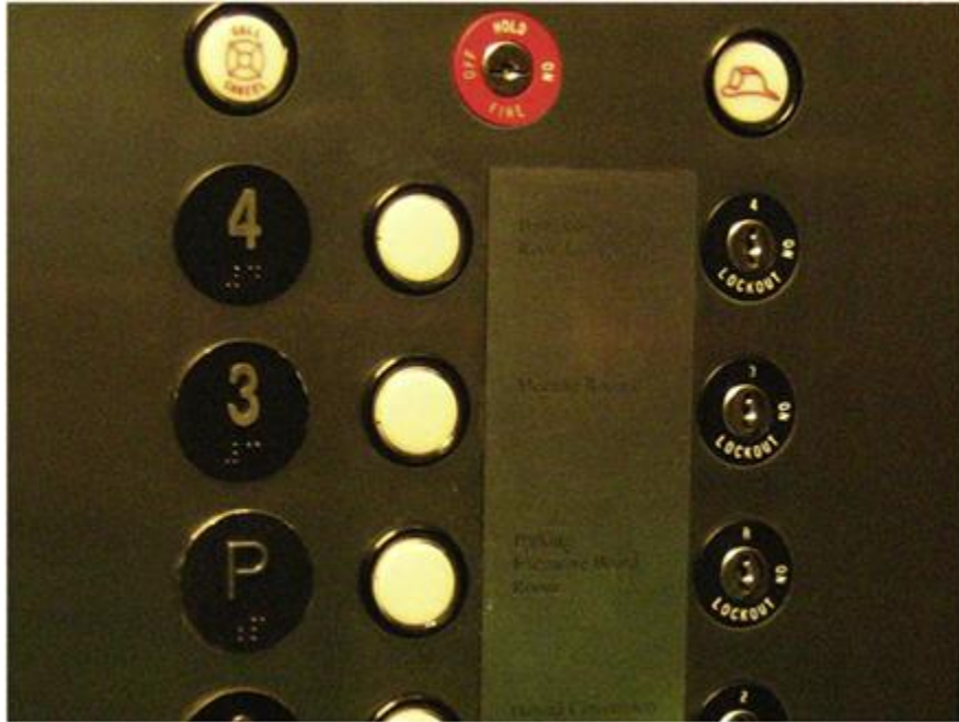
Figure 1.37 An elevator using wafer locks to regulate access to certain floors.
